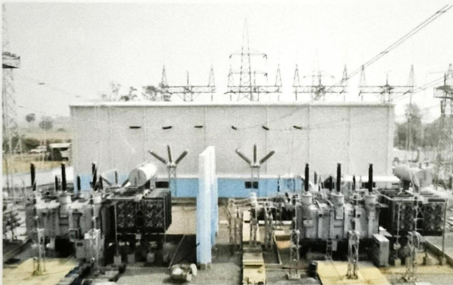
Figure: -Power Transformer
